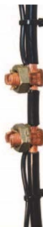
Figure 1 Example of properly terminated sensor leads. Leads are not mechanically connected, and termination points are insulated.
